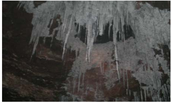
Figure 10: Hole in roof of chamber 37 and stalactites
